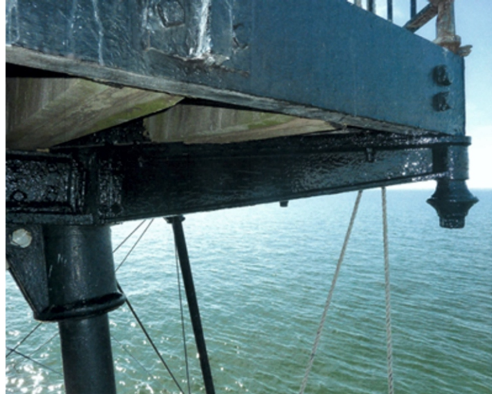
CDS coated the ancient Middle Bay Lighthouse, built in 1865, with Alocit 28:15. The structure is located offshore from Mobile, Alabama, in Middle Bay.
