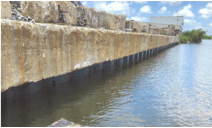
Left: Steel shipping facility ELG Metals Mobile Alabama sheet piles refaced and coated with Alocit 28:15.
