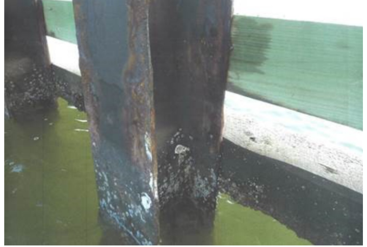
Below: Orange Beach, Alabama toll bridge blasting and coating with Alocit 28:15, before and after.
