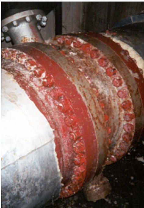
Above: 32" flange after removal of insulation showing corrosion.
